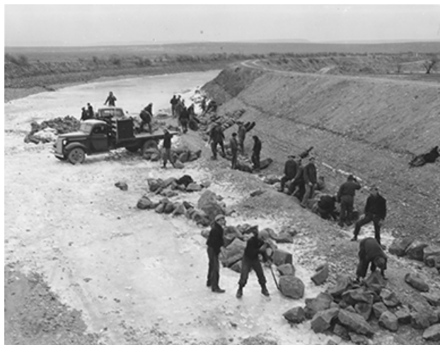
Figure 26.6 The CCC put hundreds of thousands of men to work on environmental projects around the country. Some call it the beginning of the modern environmentalist movement in the United States.
